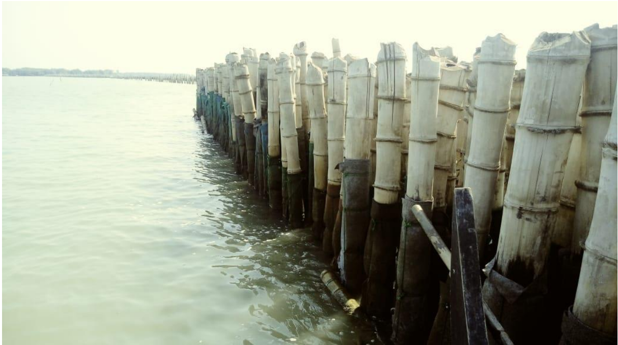
Figure 1. An application example of using a circular bamboo breakwater insulated on a muddy beach (Sulaiman, 2017).
